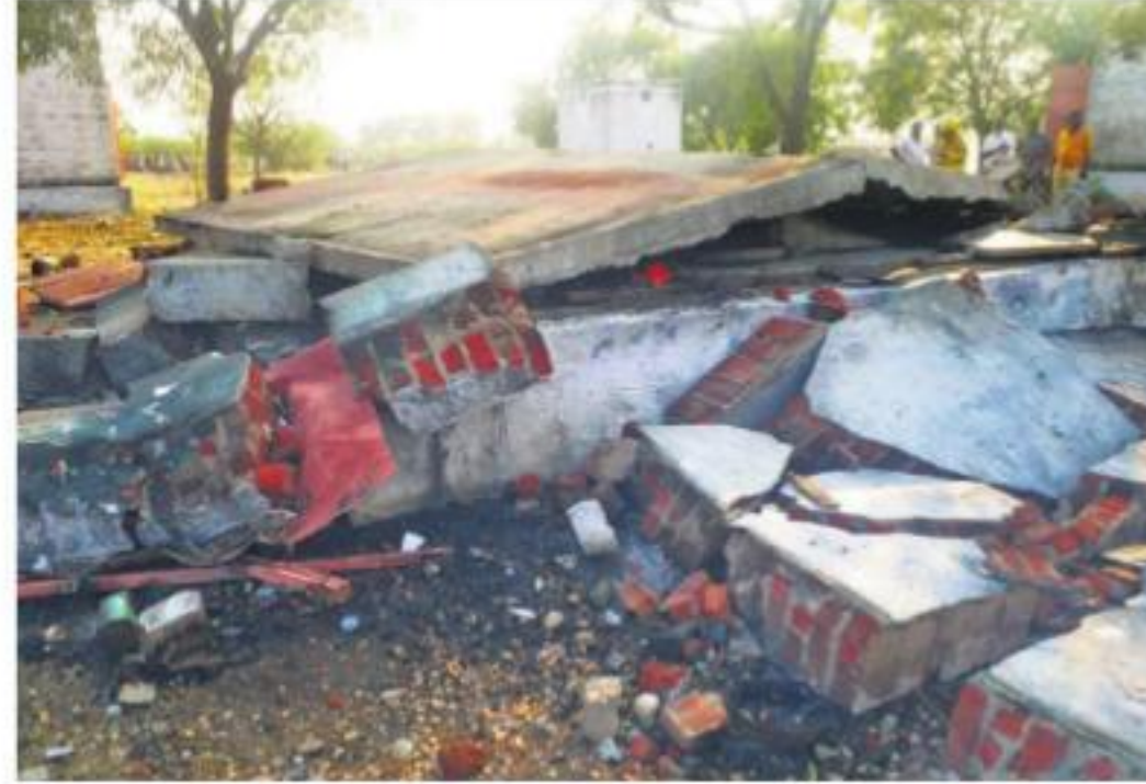
Among the 31 rooms at the cracker unit, seven got gutted and a few other rooms sustained damages | EXPRESS
