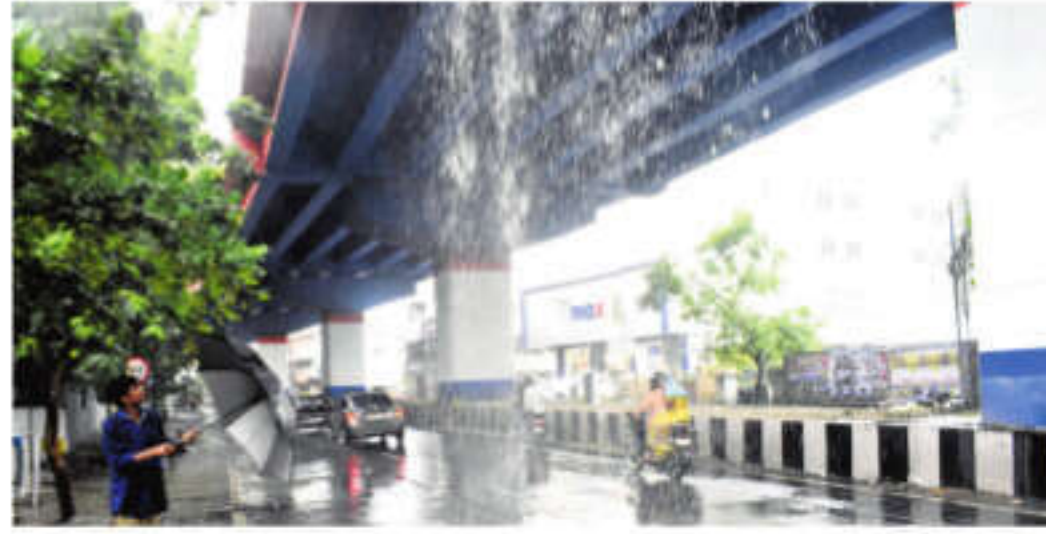
Rainwater leak from the Tiruchy road flyover in Coimbatore posing trouble to motorists and pedestrians alike | S SENBAGAPANDIYAN
