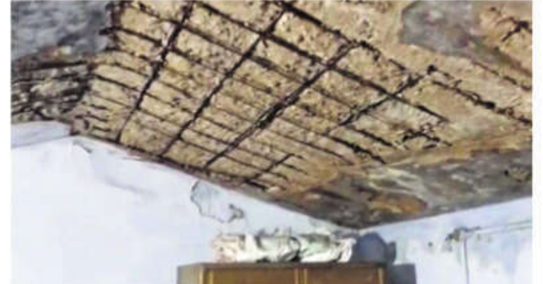
Most of the 20 houses that were built around 40 years ago for Irula people at Puliyanandi in Pollachi are in a dilapidated condition | EXPRESS
